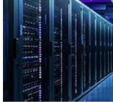
Data Center Infrastructure
