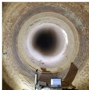
Fiber optic sensors are often used in process industry
