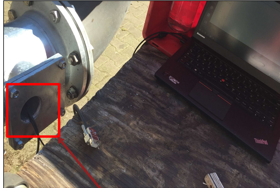
Comms cable to laptop
