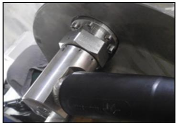
Fiber Optic Connection
